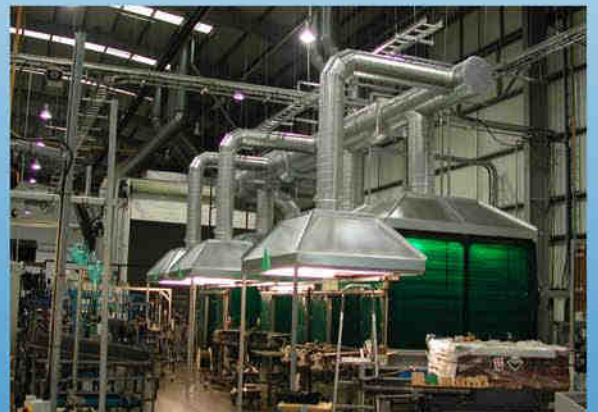
Fume Extraction System
