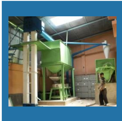
Flour Mill Besan Plant
